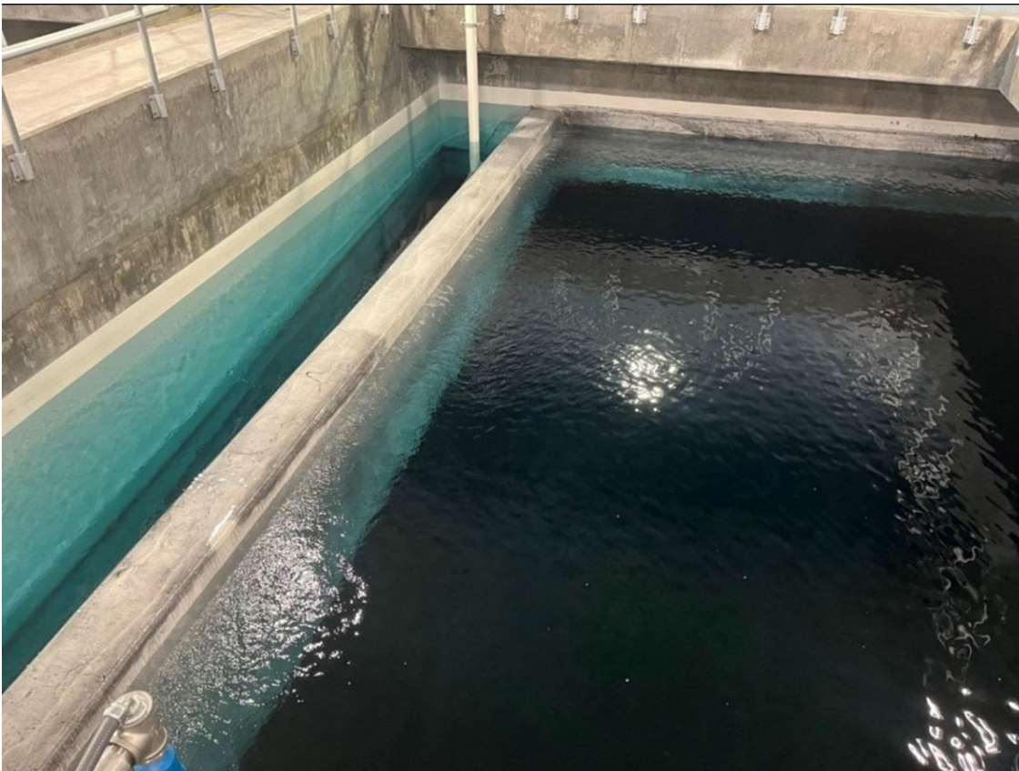
Granular Activated Carbon (GAC) media loaded into one of eight deep-bed filters at the Sweeney Water Treatment Plant.
