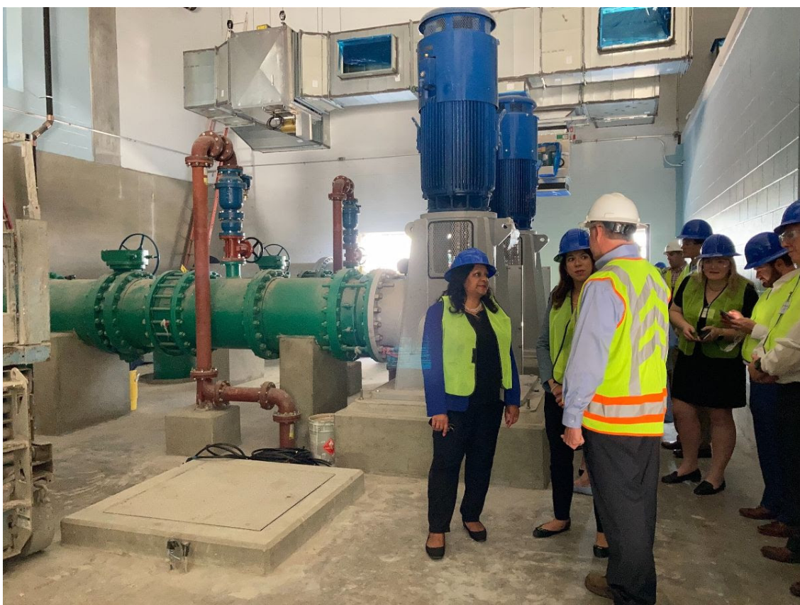
Radhika Fox, Assistant Administrator for the U.S. EPA's Office of Water, (left) and N.C. Department of Environmental Quality Secretary Elizabeth Biser (center) speak with CFPUA Deputy Executive Director Carel Vandermeijden at the Sweeney Water Treatment Plant.
