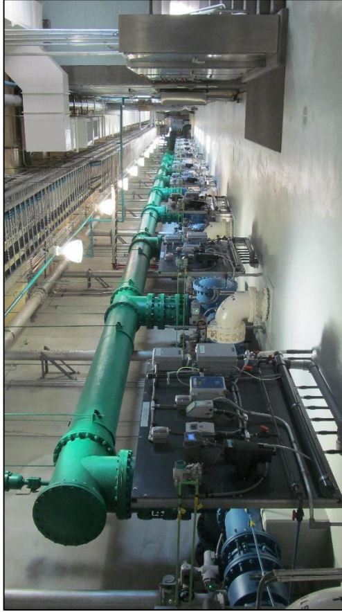
Sweeney Water Treatment Plant
