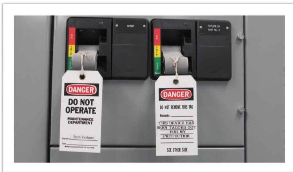
Sweeney Water Treatment Plant, photographed by Sam Yarboro
