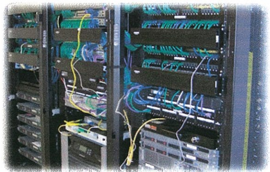
I T Communications Room
