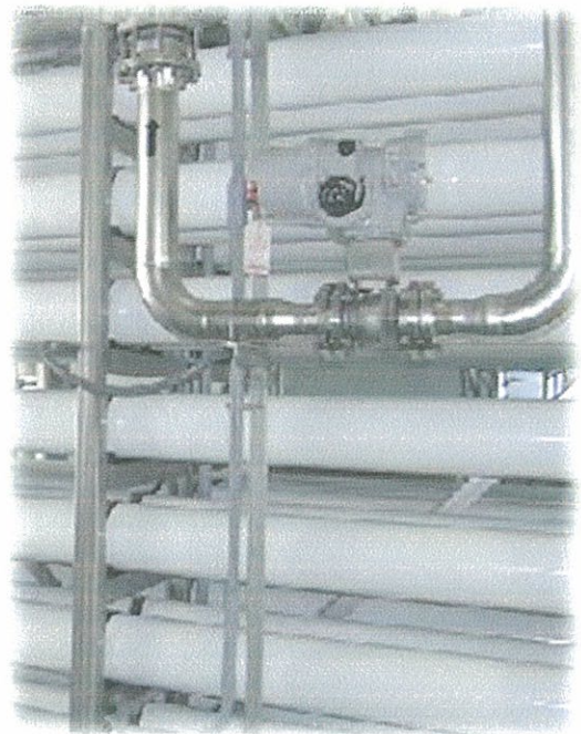
Nano-Filtration Plant Membrane Skid
